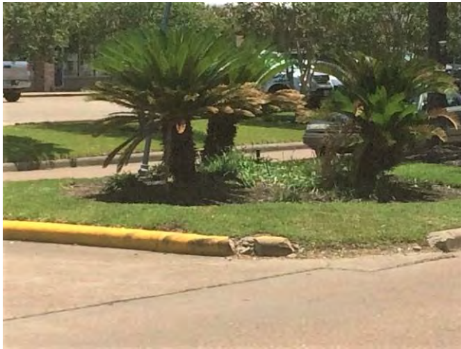
Figure 9 Broken curb in median
