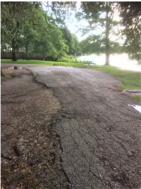
Figure 2 Founders Park - road deterioration
