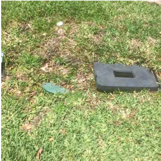
Figure 12 Water meter cover loose (East side of CVS)
