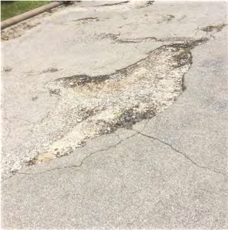
Figure 14 Frontier parking lot need repair
