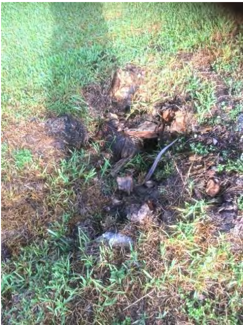
Figure 7 Spillway Bridge - 1 of 2 large holes (north of bridge)
