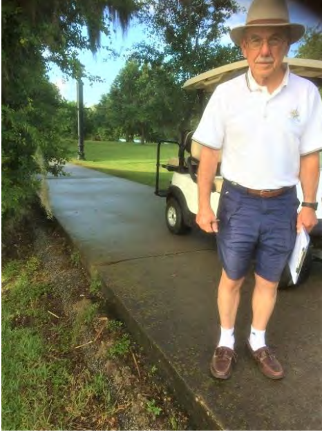
Figure 6 Spillway Bridge - Bridge walkway (North) dropoff next to sidewalk
