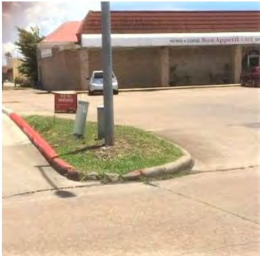
Figure 11 Broken curb at entrance to Wendy's
