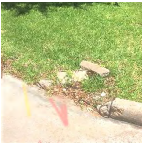
Figure 10 Broken curb in median
